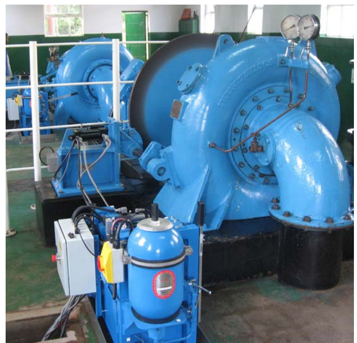
Lujeri Powerhouse after modernisation
