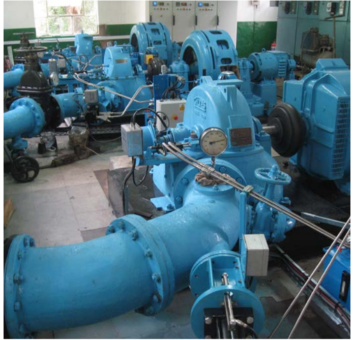
Ruo Powerhouse after modernisation
