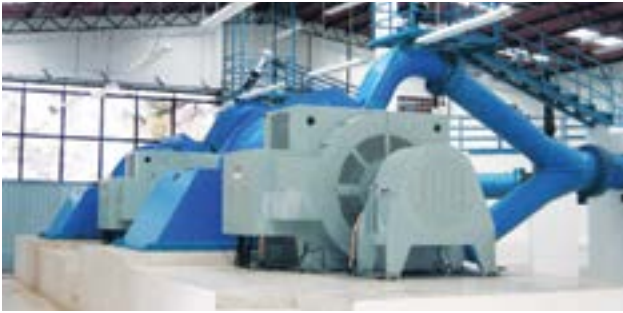
Top left: The La Esperanza project in Honduras uses twin Canyon Pelton turbines to produce 12MW from 370m (1214ft) net head
