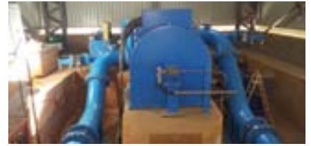
Turbine during commissioning.
