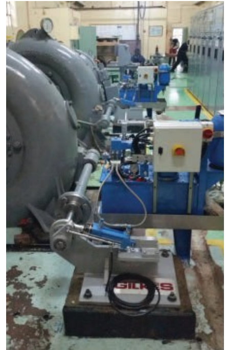
After the control system upgrade, the units generate about 10% more power and have increased operating flexibility.
