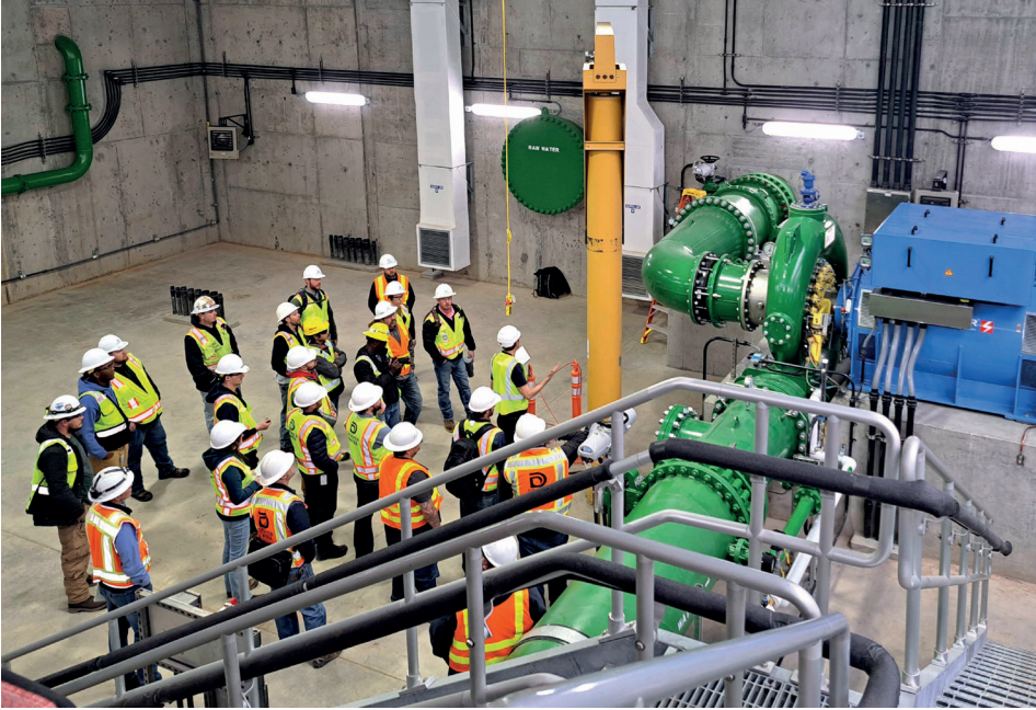
Left: Operator training during commissioning of Northwater Hydro Plant, Denver, Colorado
