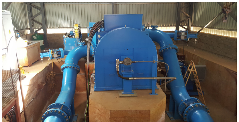
Turbine During Commissioning
