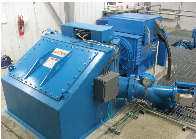
Gilkes Turgo installed.
