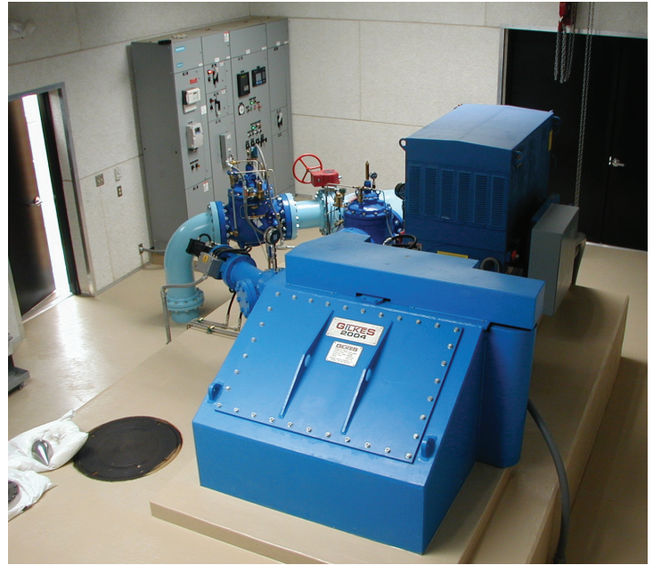
12 Inch mean diameter singlet jet Gilkes Turgo installed at Draper Irrigation Company, UT, USA. Net Head 633ft, Rated Flow 11.7cfs, Speed 1800rpm, Power 511kW, Year 2004
