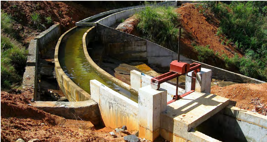
Barcaple Project Intake Sri Lanka – 1 x 2 MW
