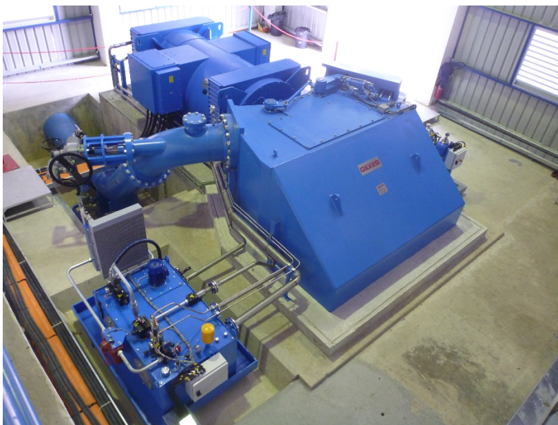
A modern 2.3MW Turgo Installation
