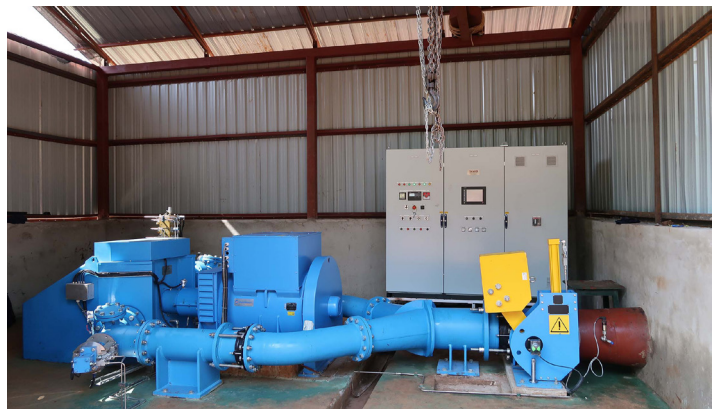
Turgo Turbine & Control Panel
